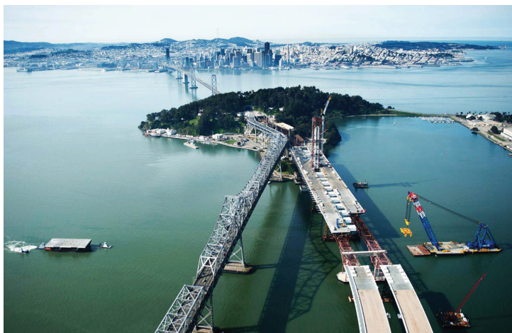
Reconstruction of the eastern section of the bridge as a causeway connected to a self-anchored suspension bridge began in 2002
